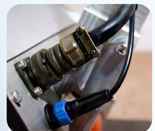
Armoured cable connectivity
